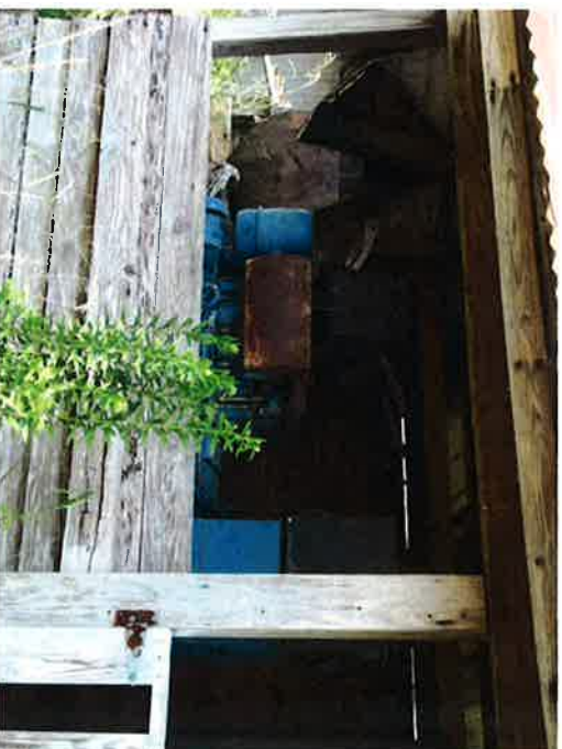
Generator shed and generator (partial view)
