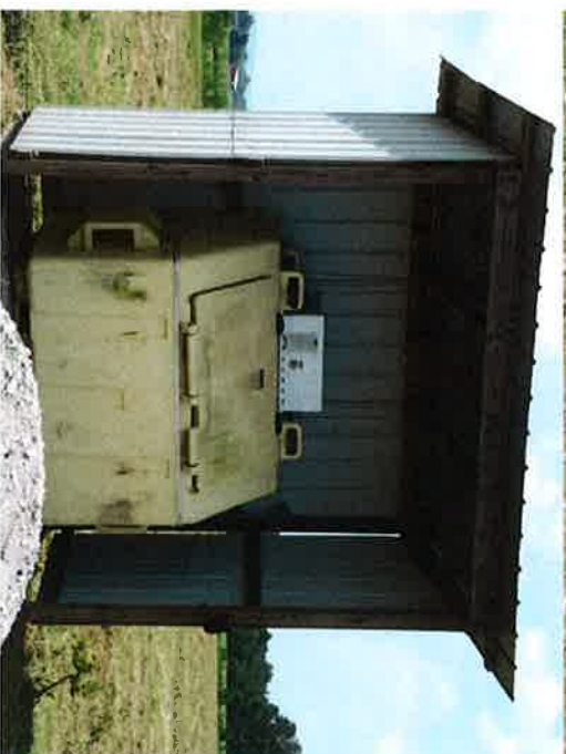
Waste disposal systems
