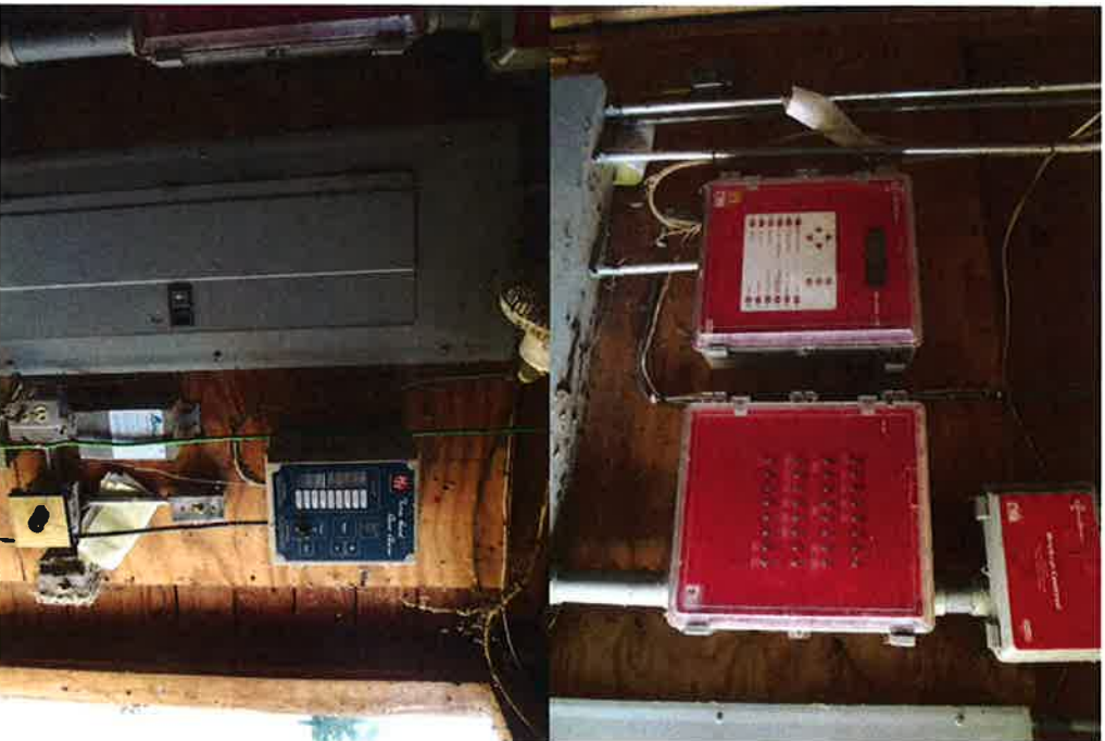
Poultry House #2 – Controls
